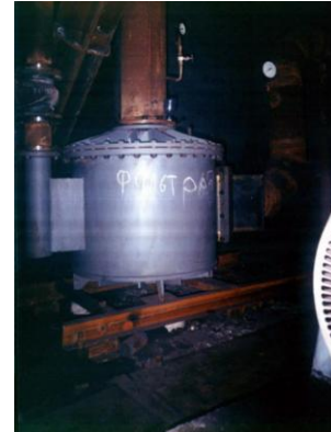
Incomplete productivity line hydrodynamic filter used utilized industrial water rectification
